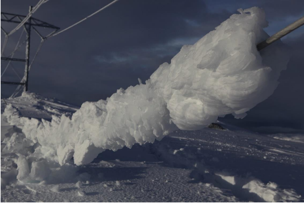
Figure 1.1: Photo of collapsed shield wire at ‘Ålvikfjellet’ 1070 m.a.s.l. in the Hardanger area, Norway, January 9, 2014. (Photo: Ole Berg, Statnett).
