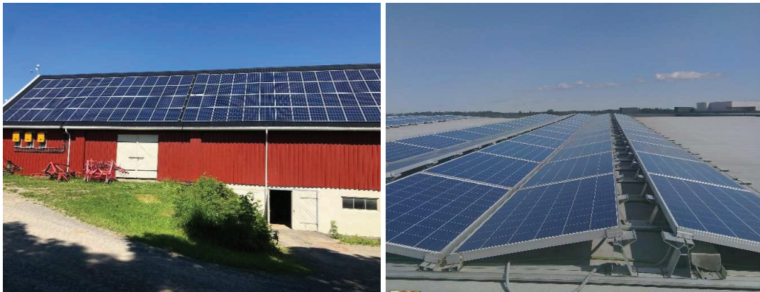
Figure 3: PV installations on tilted and flat roofs.
