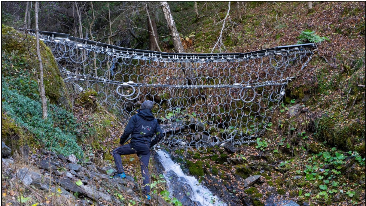
Figure 6.10 - Debris ring net installed in a historically active drainage channel near the town of Otta (Photo: Øystein Grasdøl)
