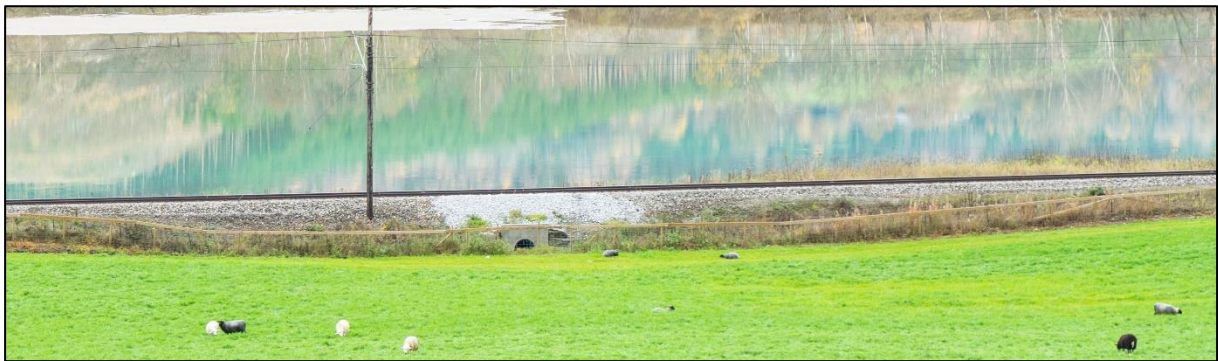
Figure 1.8 - Railway prone to flooding and debris flow in Sandbu, south of Otta. White gravel in the middle of the picture indicates a repaired section after embankment washout in 2013. (Photo: Øystein Grasdahl)
