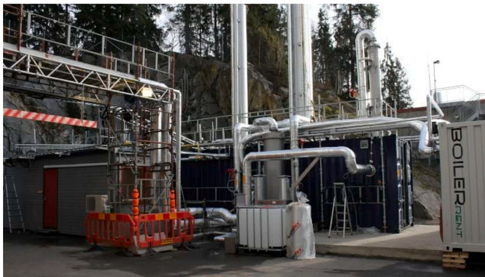
Fig. 2. 3D representation (top image (modified from FOV FEED report, 2020), container not shown) and picture (bottom image) of the FOV pilot plant for carbon capture (image courtesy of FOV).
