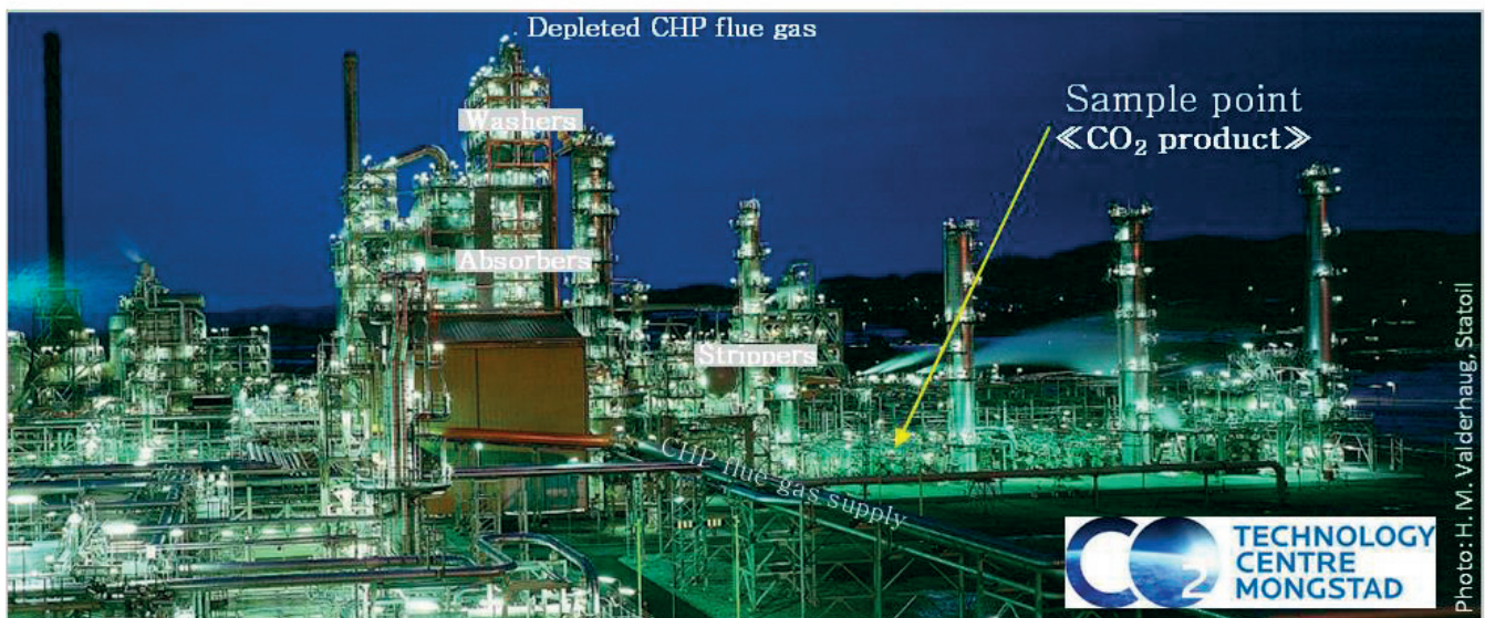
Fig. 1. Technology Centre Mongstad (TCM), Norway [Photo © Equinor] DA amine plant with CHP flue gas inlet from the front, and the high absorber tower in the middle. “Captured” CO 2 product outlet and sample point towards the right.
