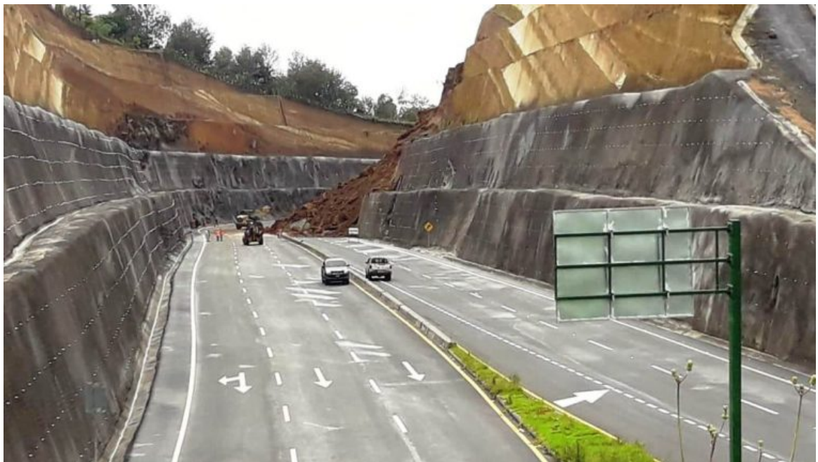
Figure: A glance at the near-vertical cuts through the earth with no structural reinforcement is enough to visualize how unsound the roadway is (the outer cement layer does little more than provide minor erosion control). It also illustrates the dramatic extent to which the earth has been carved away through what for many Maya is a living landscape. Source: Prensa Libre, Victor Chamalé.
