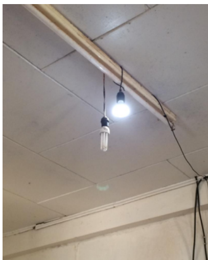
Bulbs from the new lighting system wrapped around the old tube lighting system in a patient ward. Only one of the lights was functional.
