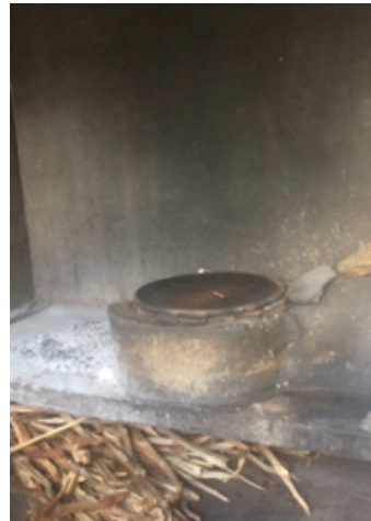
Soot on the walls in the kitchen
