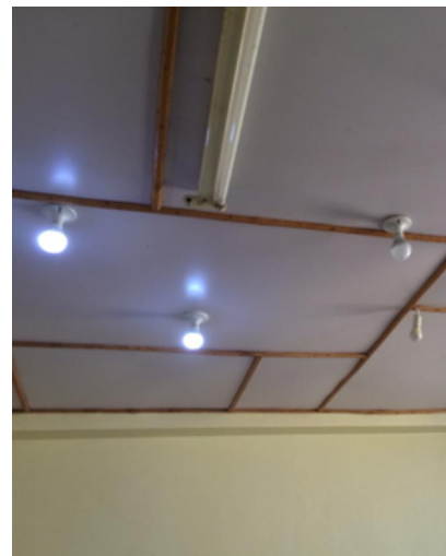
Bulbs from the new lighting system surrounding the old system in the delivery ward. Only a few of the bulbs were functional.
