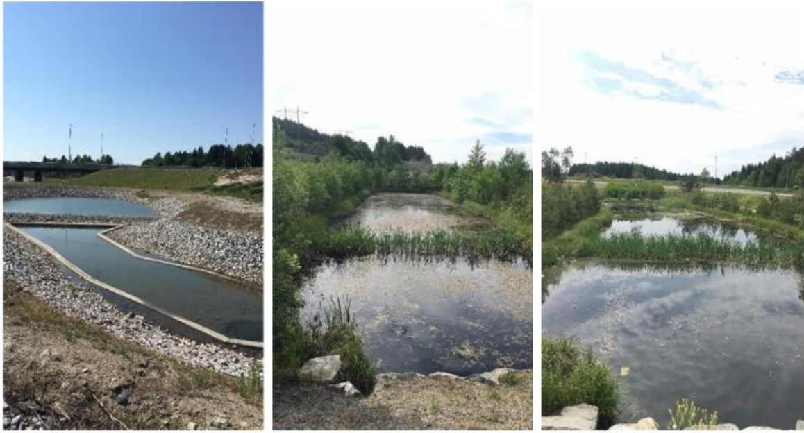
A7 – Støttum, Taraldrud North and Taraldrud Junction sedimentation pond
