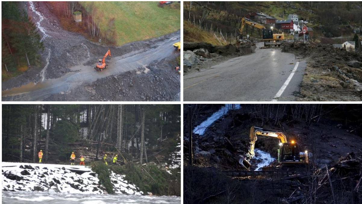
Figure 7.7: Roads (top) and railways (bottom) getting cleared quickly after landslides. All pictures were taken during “Dagmar” in 2011, except the top left, from “Hilde” (2013) top left.
