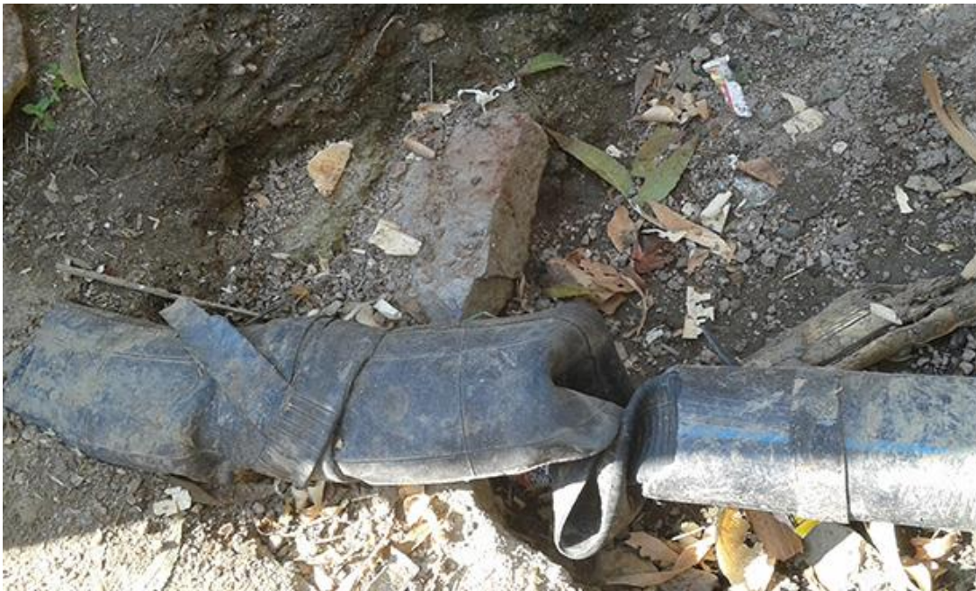
Illustration 5: Broken solar-driven drinking water pipe in Ashapura
