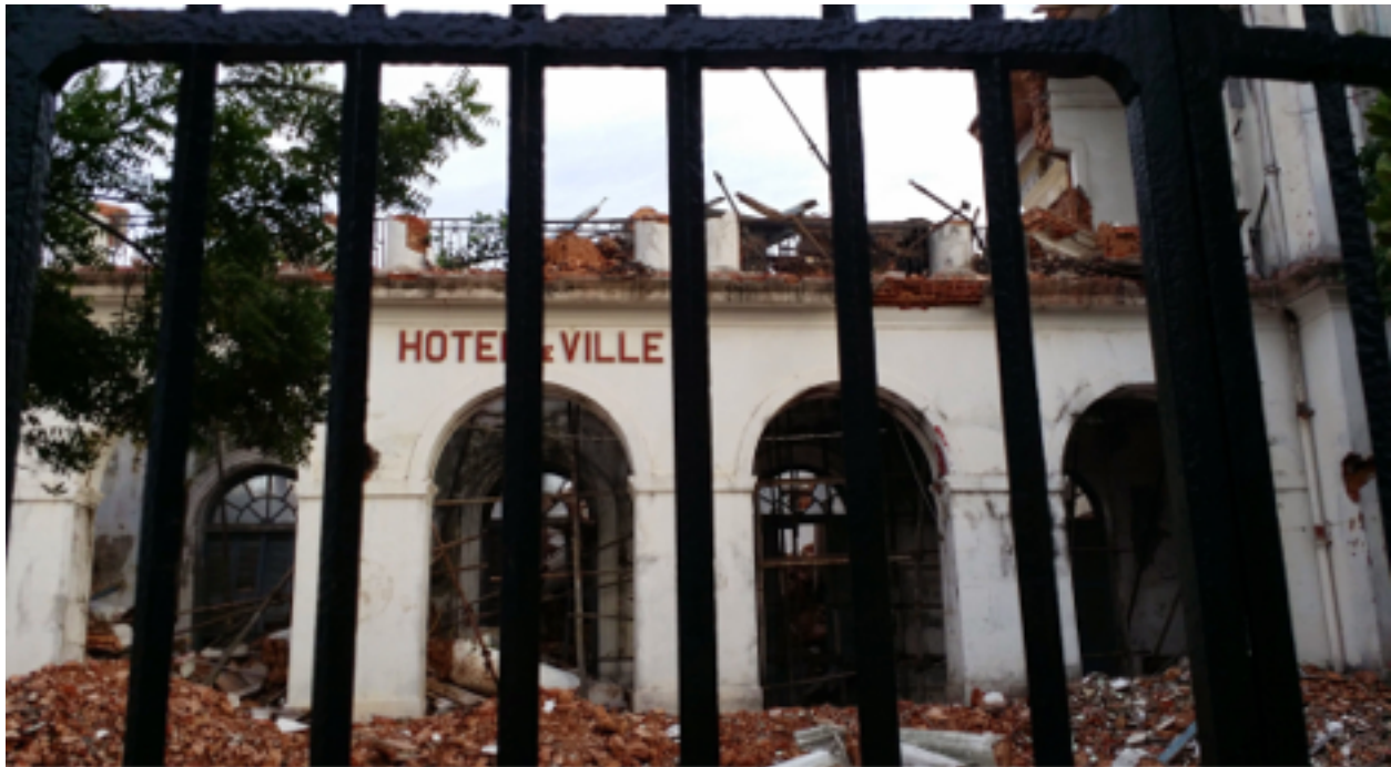
Fig: 6«Hotel de Ville - The ‘Mairie’ seen the morning after the collapse caused by the winter rain. Photo by Author
