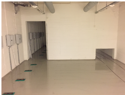
Figure 6.9: AGV charging area (green artifacts on the left)
