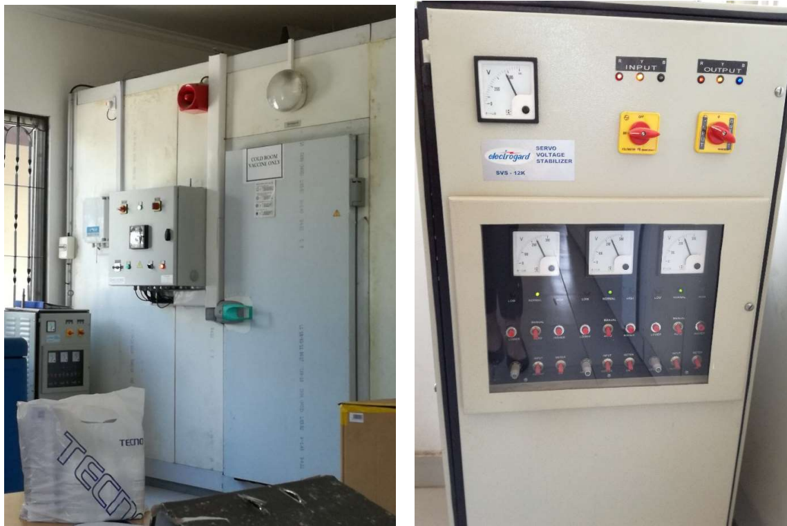
Figure 23 – “Cold room” (left) and equipment for managing its power supply (right)
