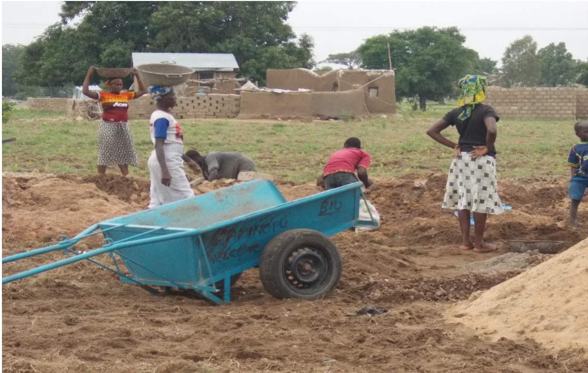
Figure 5: The cement house building site of a contract farmer. Source: Fieldwork July 2014.
