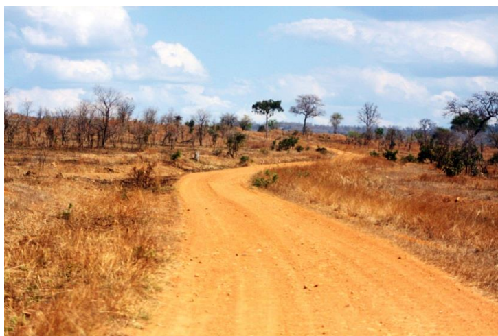
Figure 6.1 – Example of poor road infrastructure
