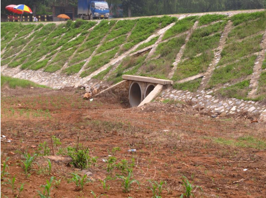
Figure 18 Flood dam in the low land area in the south shore of the reservoir (photo: Ellen Pettersen).
