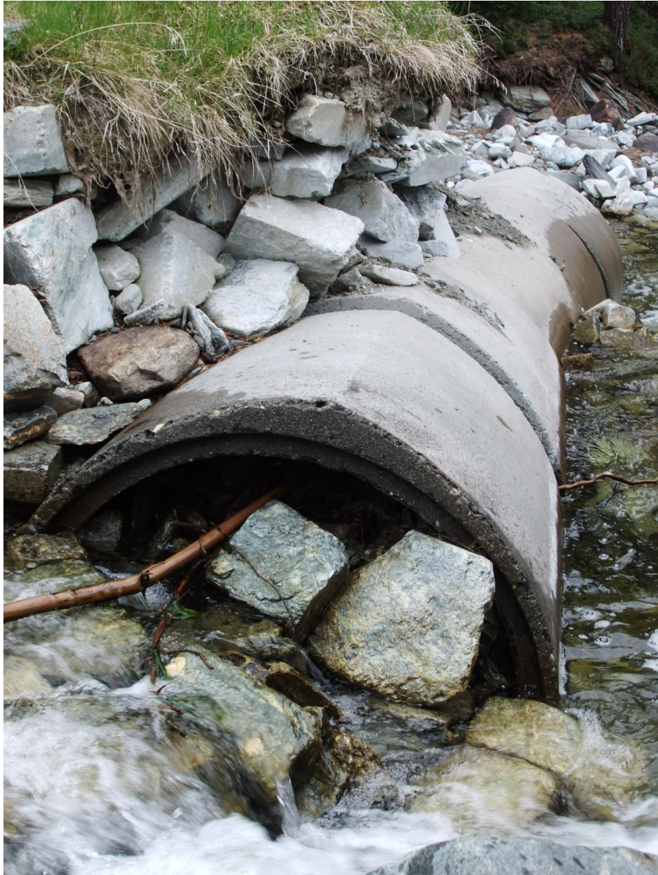
Figure 4.3.3 The totally blocked drainage pipe for the second bridge.
