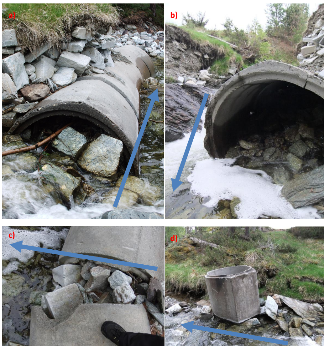
Figure 5.3.2.7 a) the front side of the five tubes; b) the back side of the five tubes; c) the middle of the two tubes being flushed away 4-5m away; d) the furthest tube being flushed away.
