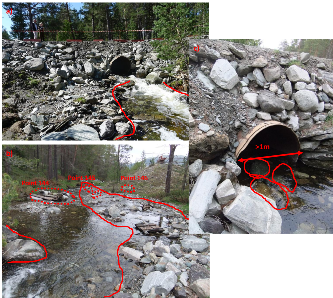
Figure 5.3.2.1 a) the repaired bridge; b) the open field after the failure point, circled by the red dash line showed the flushed concrete pipes. Area circled by the red solid line in a) and b) showed the debris deposits behind the bridge.
