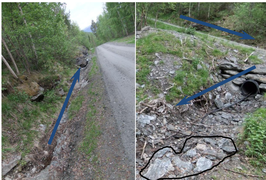
Figure 5.2.2.1 Main road of the location and the drainage pipe in the start point. Blue arrows show the declination of the slope and the flow direction in the channels, and mineral shale showing in the second figure in the black circle.
