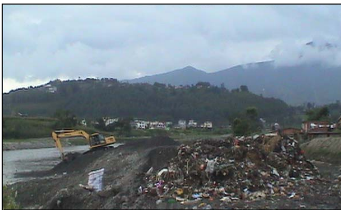
Plate 4.7: Bagmati River, ditch making at the bank and pile of waste ready to bury
