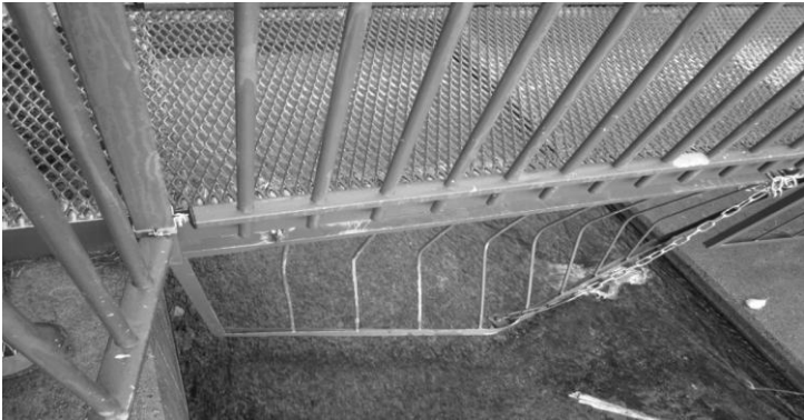
Figure 2.15: Damaged spillway of Årbogen dam, Norway (Pictures from site visit with NGI on 28 th October 2010)
