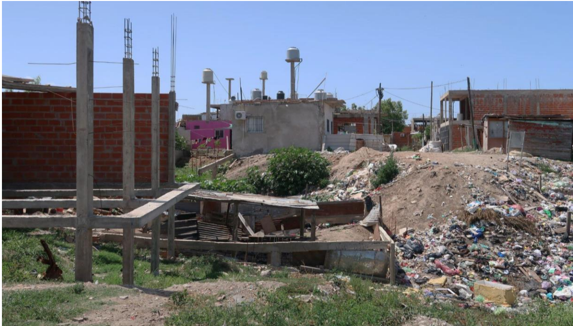
Figure 107. Foundations for a new house are laid at the same time as the land is being elevated and filled with garbage.
