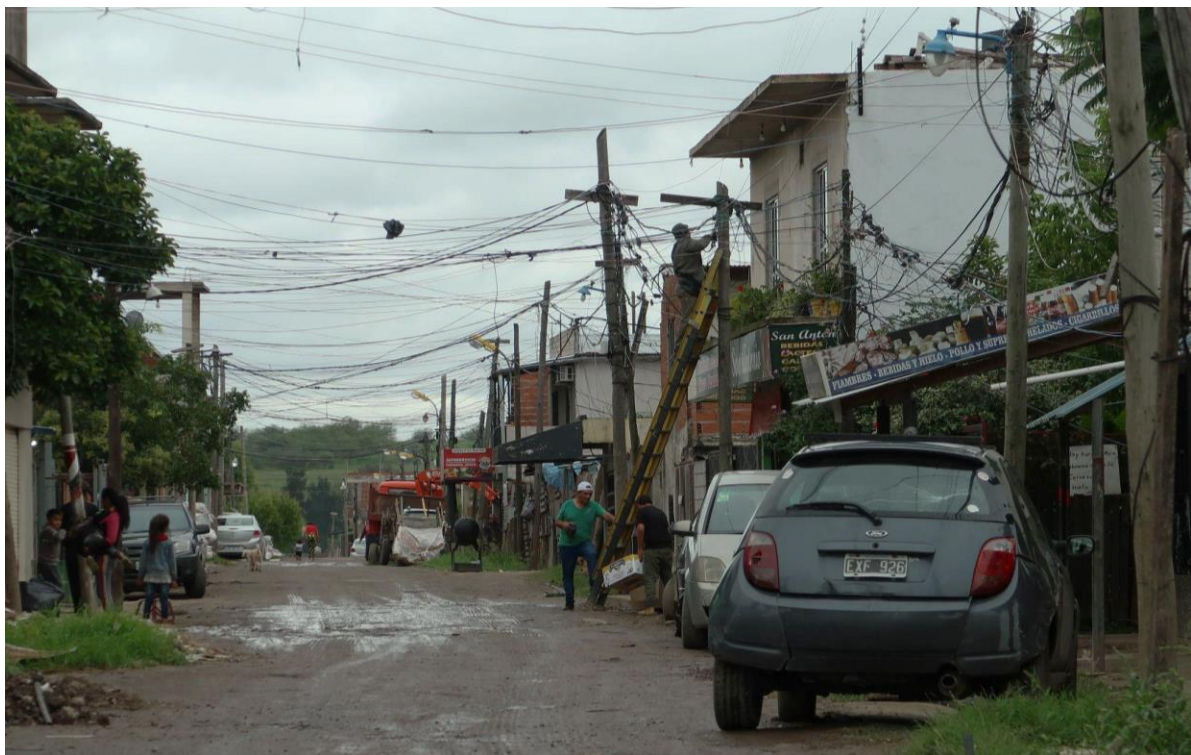
Figure 109. Informal maintenance of electric connections.
