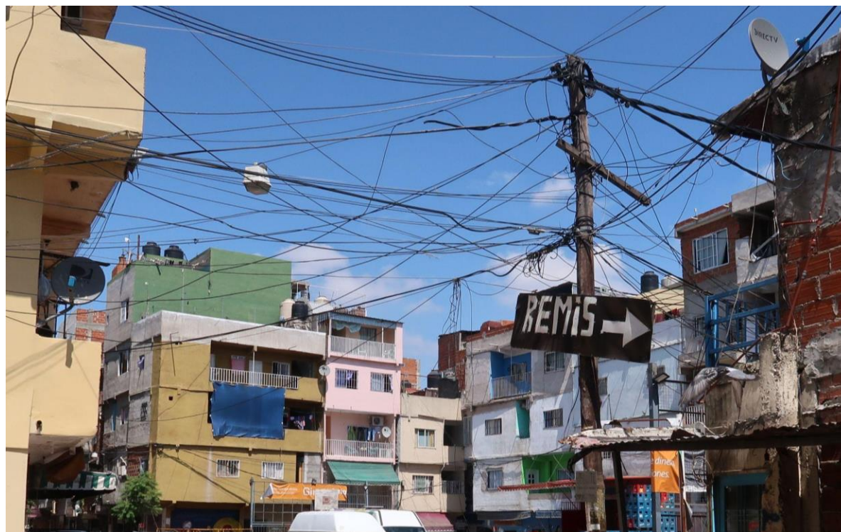
Figure 28. Hanging electric wires in Villa 1-11-14.
