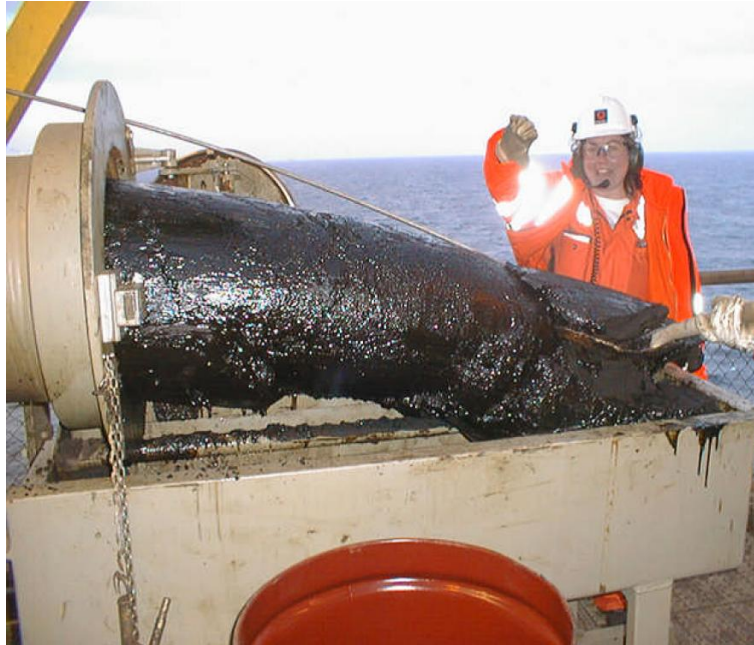
Figure 1.1: A completely blocked pipe from the Norwegian shelf
