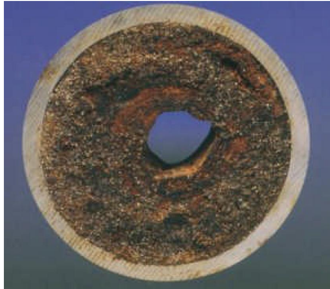
Figure 1.2: Wax almost blocking the pipe
