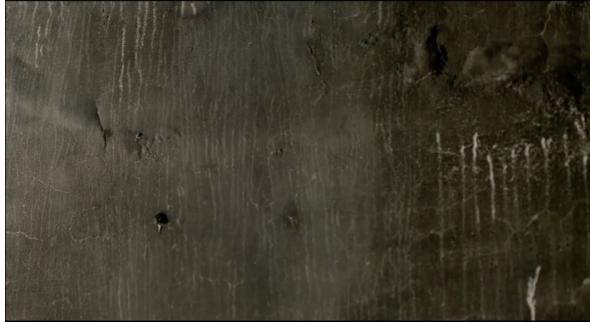
Fig. 9 Stray Dogs : A close-up of the texture of the burnt house walls
