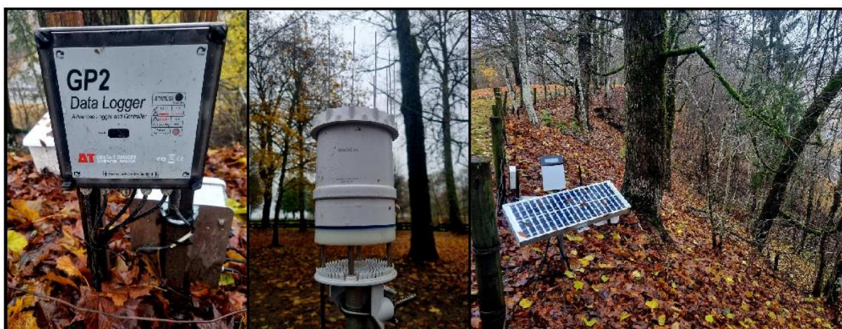
Figure 4-12. Pictures of the installed instruments. Left: The Delta-T GP2 datalogger. Middle: Atmos 41 local weather station. Right: Solar-powered 3G/2G Modem Gateway. (Photos taken during visit to the slope 3.11.22).
