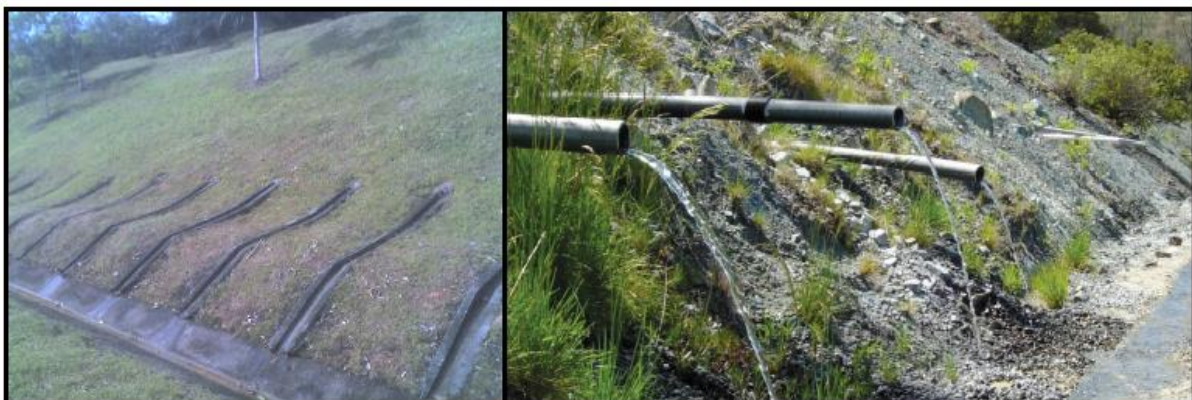
Figure 4-15. Left: Shallow surface drains. Right: Horizontal subsurface drainpipes for landslide prevention in road construction (Chatwin, 1994).
