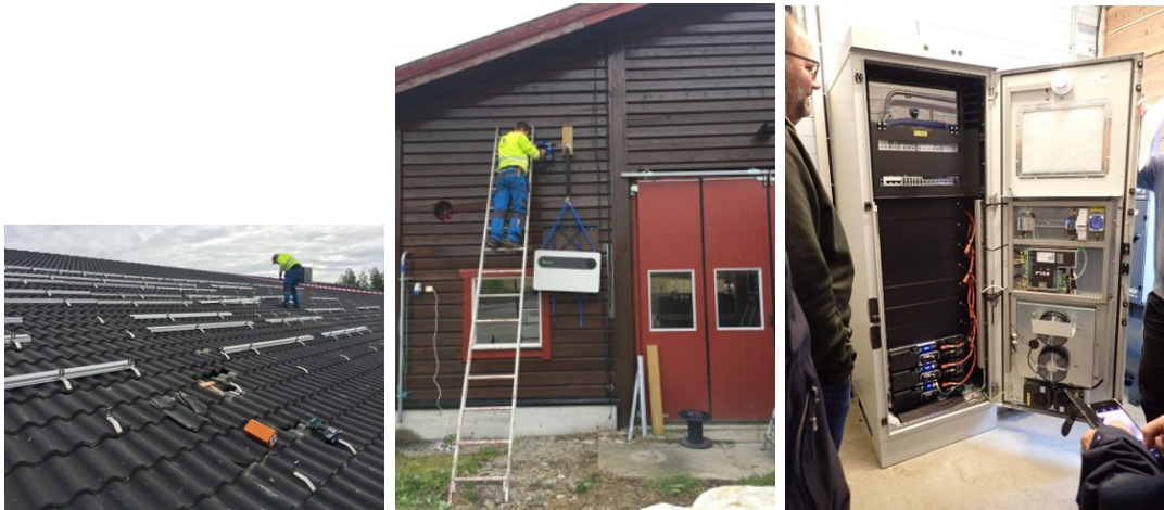
Figure 3.1: Pictures of the installation of BESS and PV on a farmhouse in Bjorkelangen. Source: Solcellespesialisten AS
