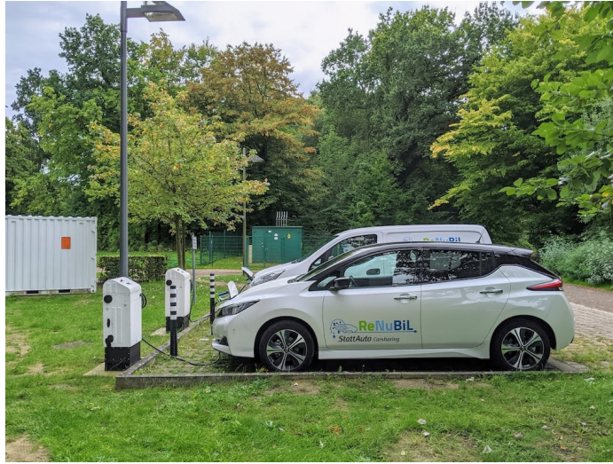
Fig. 1. ReNuBiL living lab on University of Lübeck’s campus with two electric cars, two bi-directional charging stations, and stationary battery container
