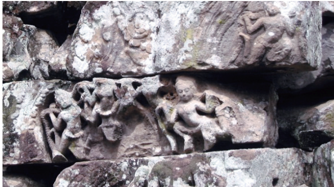
Figure 5.1: This rock art on Angkor Wat has been damaged due to salt crystallization. The white substance on the surface of the rock is so-called efflorescence, where salts have crystallized on the outside of the rock. Crystallization is more damaging if it takes place in pores within the rock, so-called subflorescence, and this has resulted in fracturing and scaling. Whether efflorescence or subflorescence takes place is largely controlled by transport processes.
